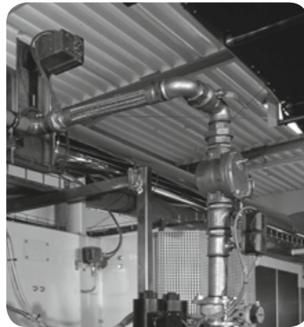
Stainless steel flexible tubes in the supply lines of buildings
