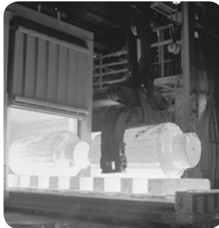
Bogie hearth forging furnace in the metallurgical industry
